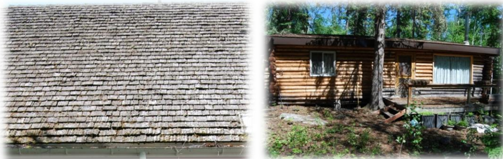
Figure 1: (Left) Wooden shake roof with needle & twig accumulation within rain eaves trough and on roof surface. (Right) Softwood conifers left too close to cabin with dried tree needles and debris on roof, deck not skirted.
